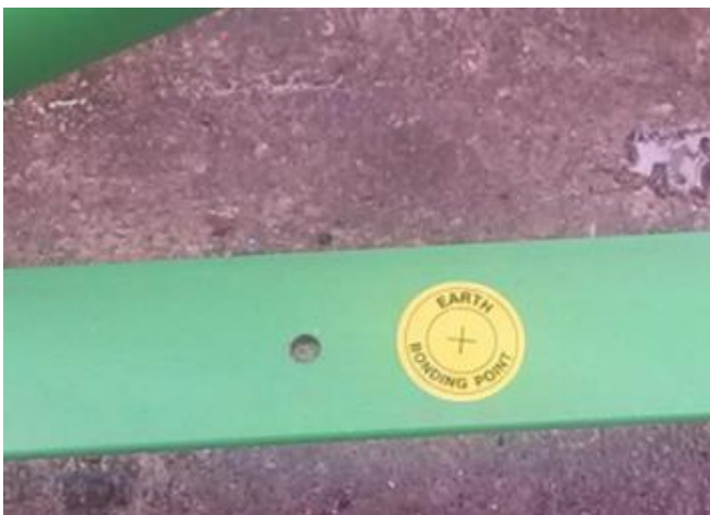
Figure 1: Earthing point marked by manufacturer
