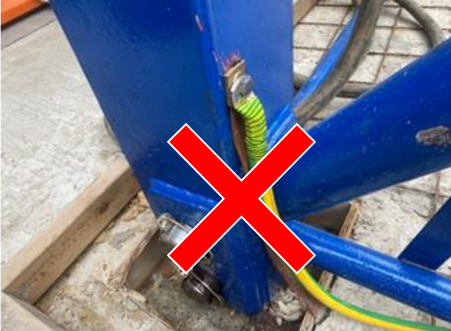
Figure 2: Earth incorrectly connected to a non-manufacturer approved point. The structural member should not have been drilled and tapped as this could weaken the member.
