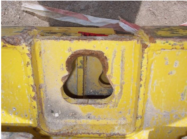
Figure 1 - Heavily burred lifting point
