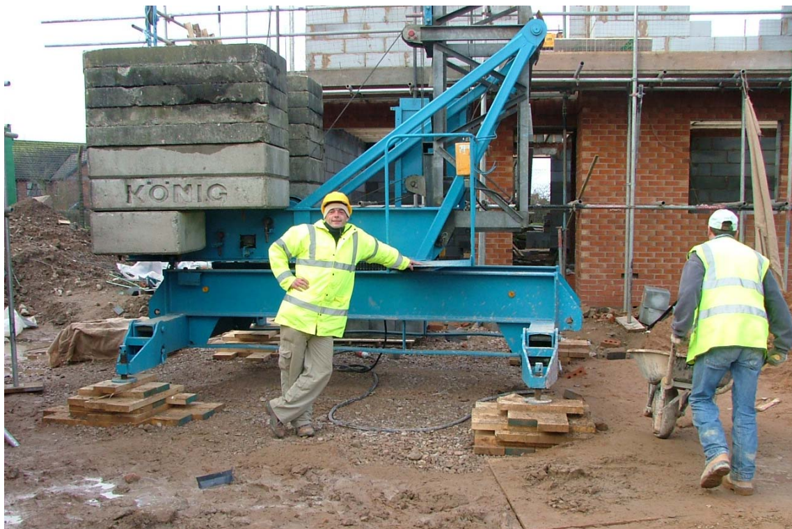
Lack of base fencing (See 5.2)
