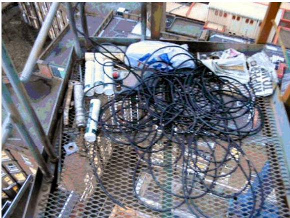
Figure 1 – General Loose Material
